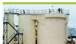
Densadeg® steel structure
