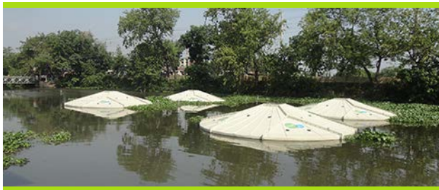
Surface aerator in canal
